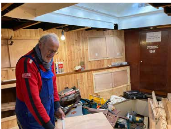
betimmering in messroom/achterin
